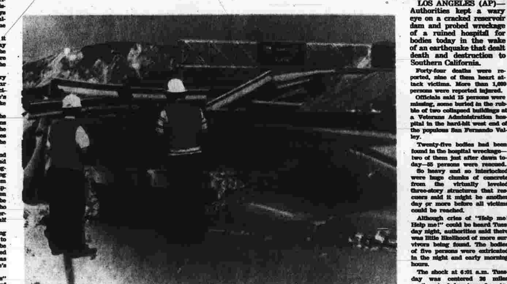
Highway crews inspect damage on Golden State Freeway, near Sylmar, west of the San Fernando Valley. Collapsed overpass is in the background. (AP Photo)
